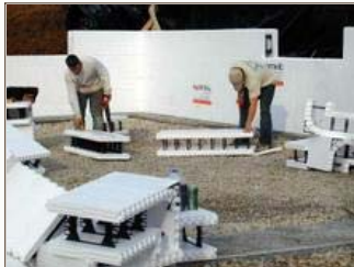
Provided by Dick Kuhn Workers cut LEGO-like pieces to fit in the wall of a home under construction. The pieces — Insulated Concrete Forms — have steel rebar in the middle, and will be filled with concrete.
